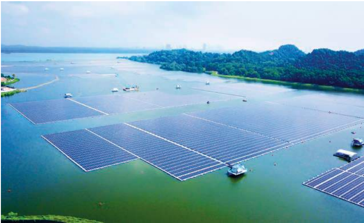
The Sembcorp Tengeh Floating Solar Farm is one of the world's largest inland floating solar farms Photo courtesy of Sembcorp
