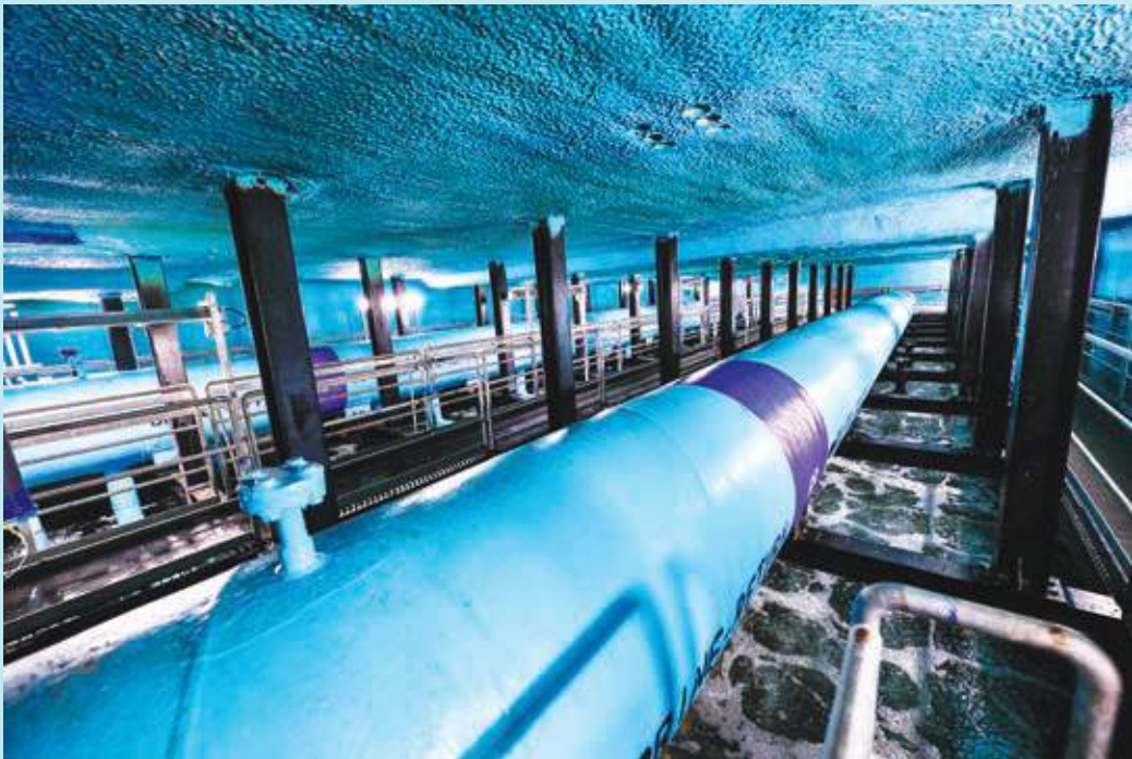
The Marina Bay district cooling network has achieved zero downtime since operations began in 2006 Image courtesy of SP Group
